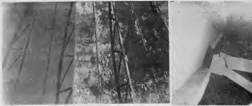
The most effective anti-corrosion paints are consistently being sought. Shown above is the interior roof of a spherical where point tests were made. While the tank was out of service, various points were sampled at different parts. Later, after the tank had been in service, E.I.G. men compared the satisfactory result at left with the best painting at right.
